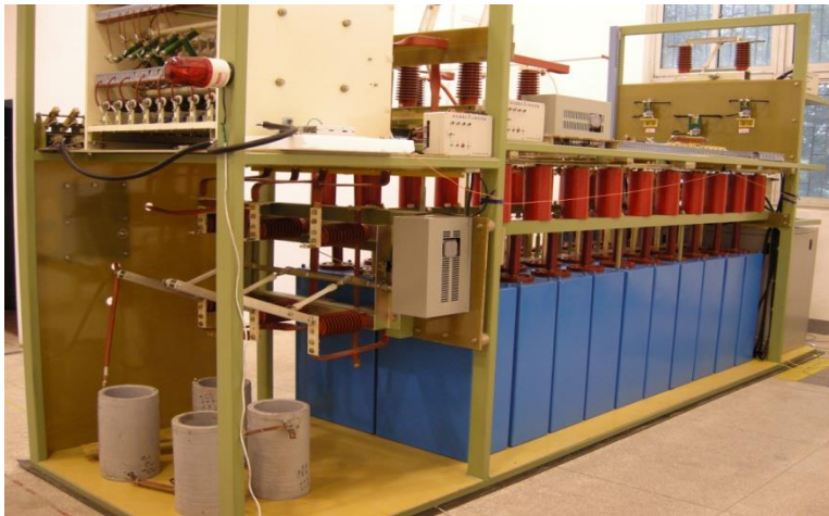
Fig.1 1MJ/25KV pulsed power supply
